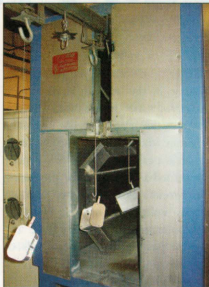
An overhead conveyor carries powder coated parts from an electric infrared system.
